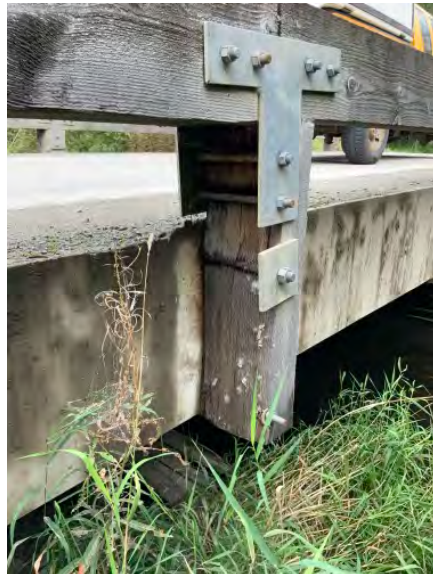
Guard Rail post damage downstream right side
